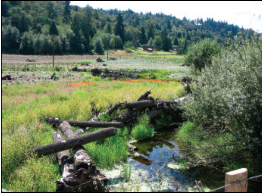
Log jams were constructed at key locations to protect the banks of Evans Creek from increased flood flows.
