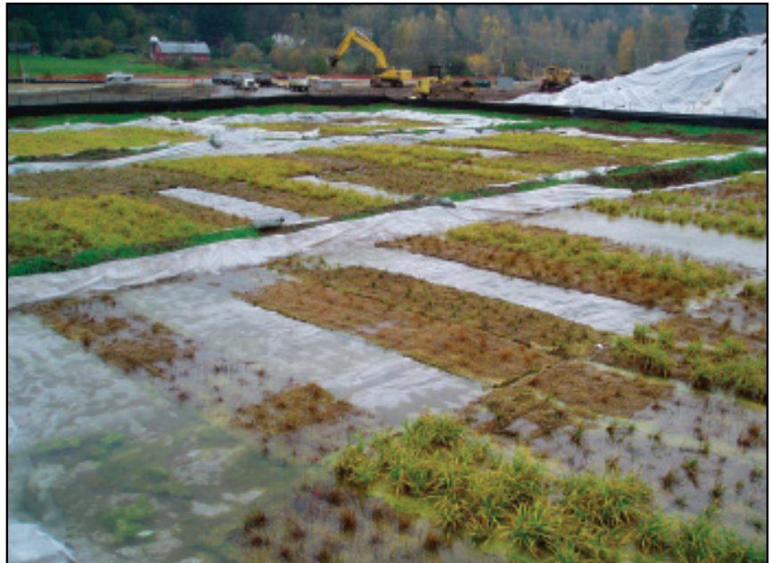
Temporary wetland sod mat paddies were constructed to stockpile the sod prior to use and during winter.
